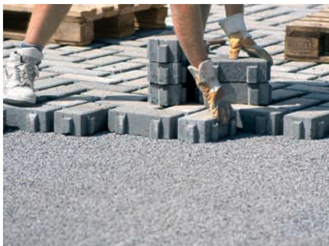
Fig. 45: Composite stone pavement with grass joints for a parking roof on top of a gymnasium.
