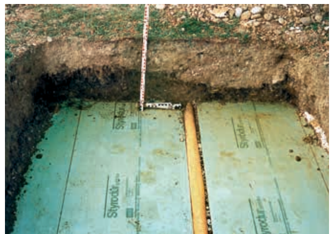
Fig. 6: Image shows a green inverted roof that is more than 30 years old
